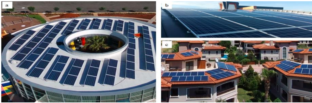
Figure 1: PV panel roof applications; a) terrace roof PV systems, b) integrated PV systems, c) mounted PV systems (Daima Enerji, 2023).
